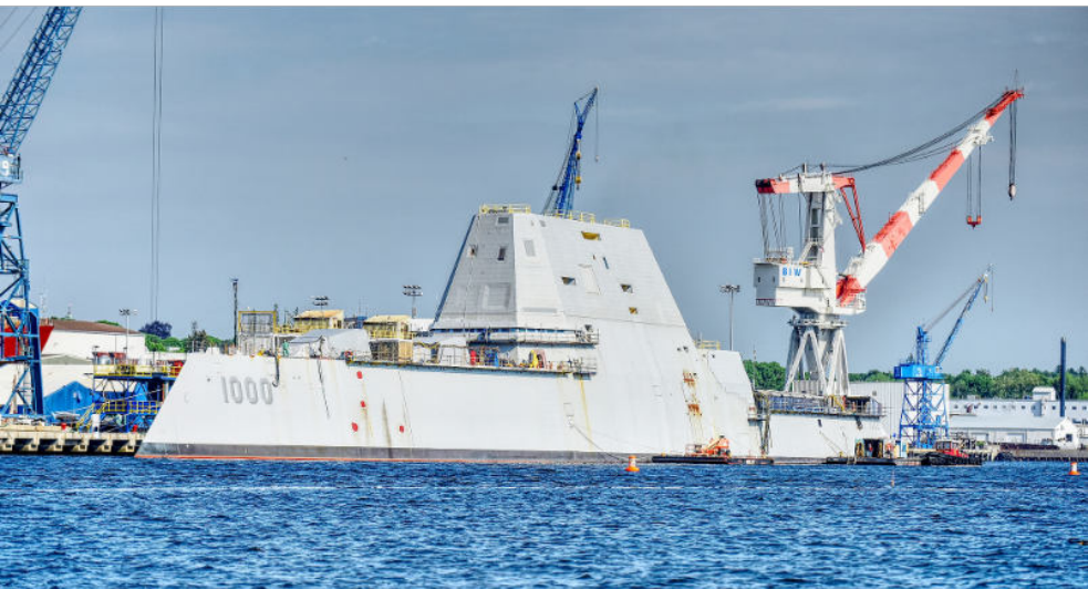
A Zumwalt-Class destroyer being built for the U.S. Navy at Bath Iron Works in Bath, Maine.
